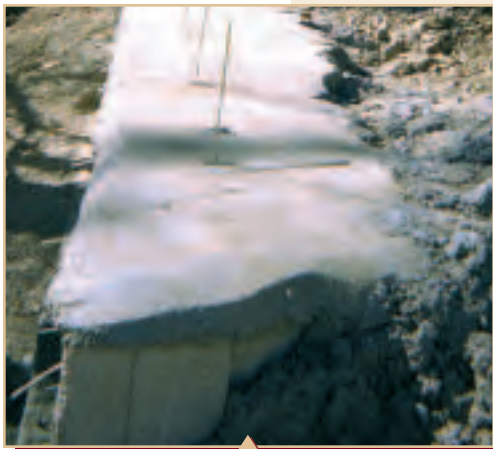
View of top of wall elevation showing grouted cap serving two purposes: (1) seal off water (2) secure wire to units and provide clean surface for rock attachment.
