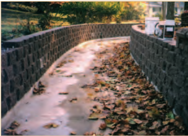
Keystone was chosen for a drainage ditch improvement project by the City of Manassas, Virginia.
